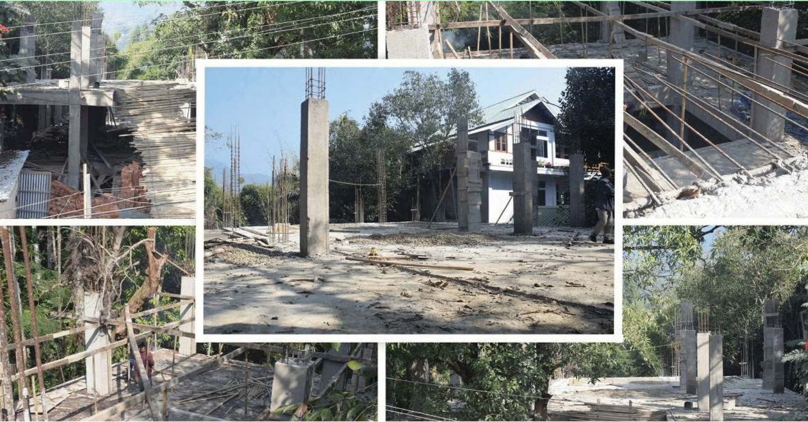
CONSTRUCTION OF TRIBAL MUSEUM IS UNDERWAY AT KAMALANAGAR UNDER MUSEUM GRANT SCHEME, MINISTRY OF CULTURE, GOVERNMENT OF INDIA.
